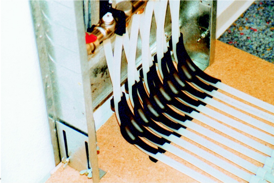
The plastic bend supports are a perfect guide for the tubing at the manifold box
