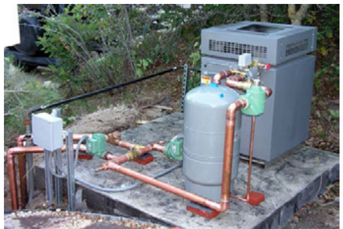
Pictured above is a snowmelt boiler system designed to be placed outdoors. Weather-proofing must be considered in the design application of this system. This is a great option for when indoor space is not available.
